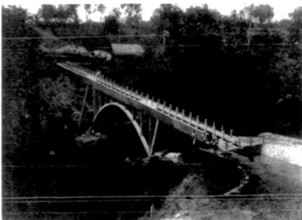
The aqueduct at Tanah Djawah that was built in connection with the waterworks at Simeloengoen.
